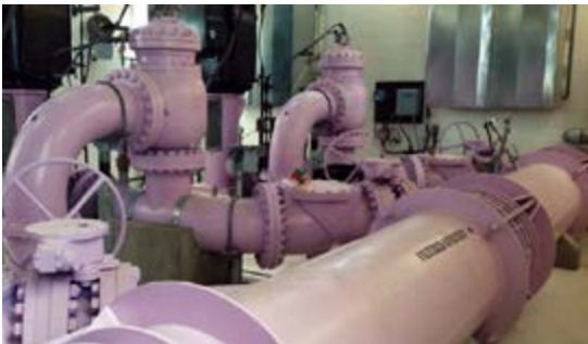
Caption: Purple pipe that moves non-potable water.
