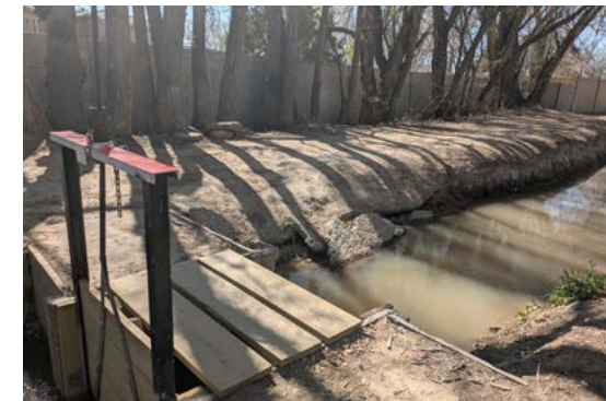
Caption: Headgate located on the Griegos Lateral
