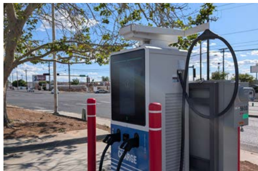
Caption: Newly installed EV charger near Montañó Boulevard and Edith Road.
