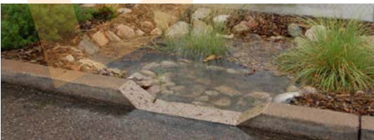
Caption: An example of a curb-cut as Green Stormwater Infrastructure.
