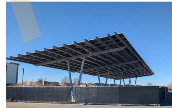
Caption: Photovoltaic covered EV Chargers at Avanyu Plaza at the Indian Pueblo Cultural Center
