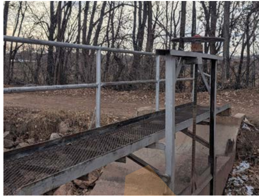
Caption: A headgate along Duranes Lateral.
