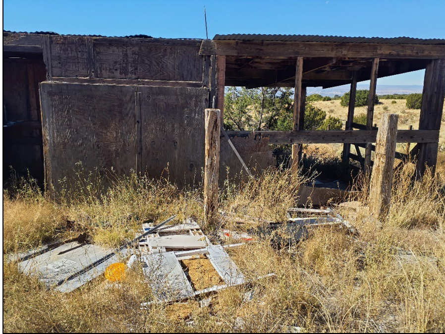
Figure 5. Overview of recent building within survey area, recent corrugated roofing and metal joist hangers, associated trash in foreground, facing south (Frame -0962).
