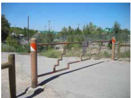
26. Pipe Gate with Pedestrian Opening
