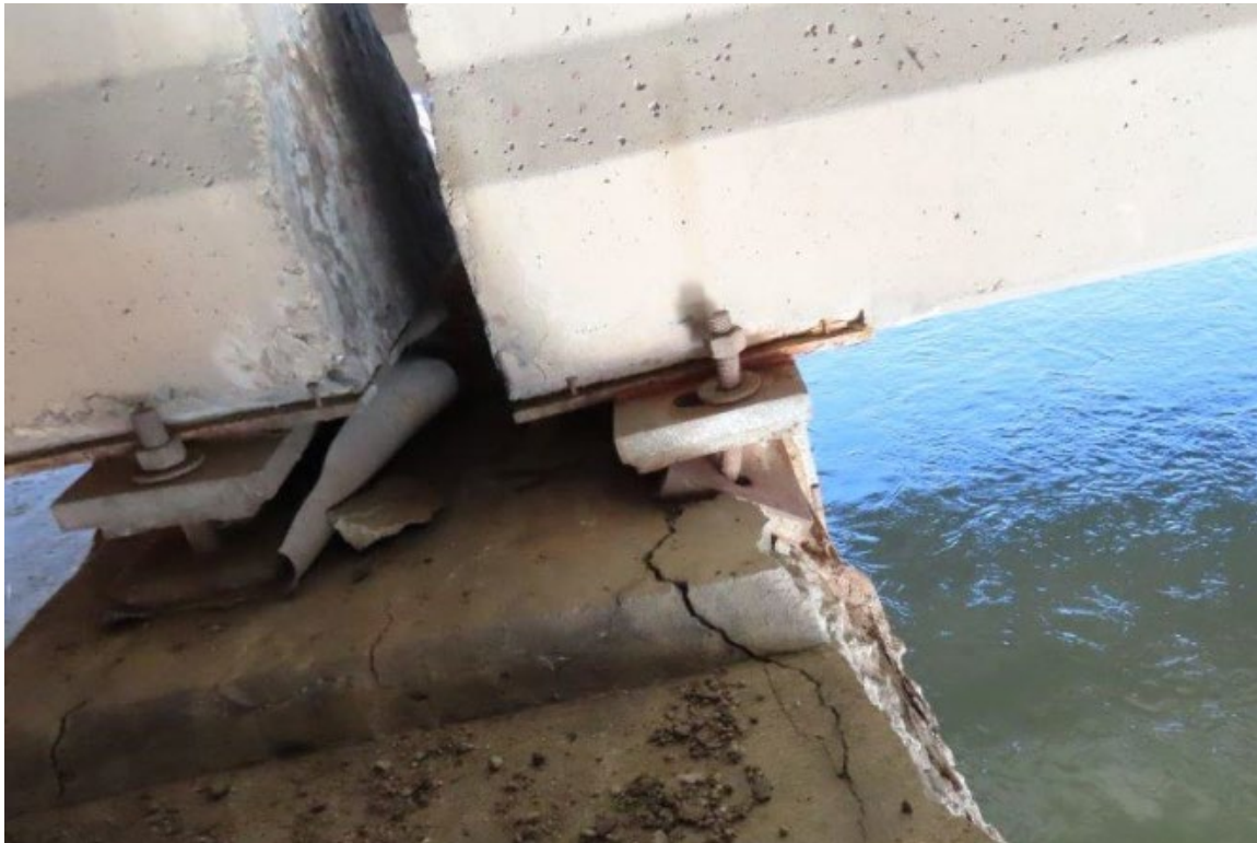
The Damage (Before)
