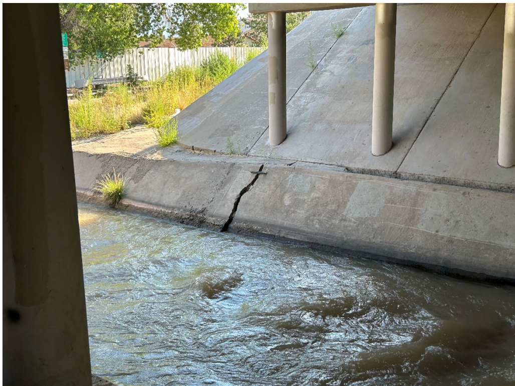
Figure 13: Condition of the bridge over the Albuquerque Riverside Drain.
