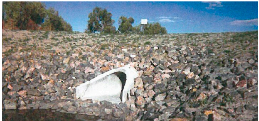
FIGURE 6.10.28 Unprotected Culvert Outlets Cause Downstream Erosion
