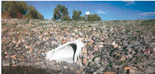
FIGURE 6.10.28 Unprotected Culvert Outlets Cause Downstream Erosion
