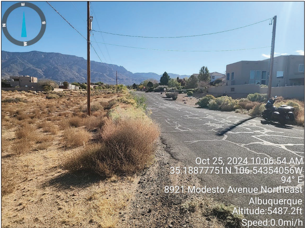
Figure 3 - Lack of Sidewalk on Modesto Ave NE
