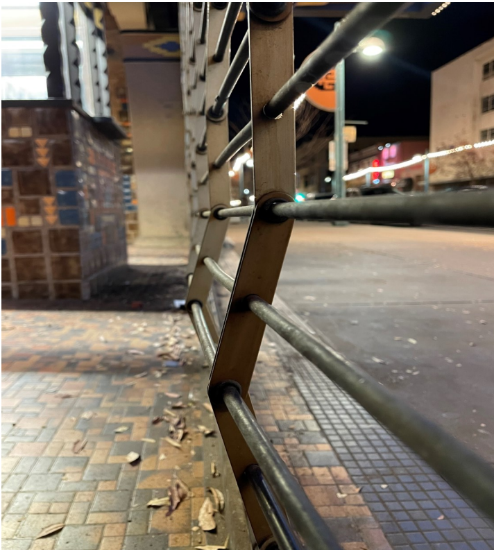
People leaning and pushing on the grill repeatedly have made it bent and broken.
