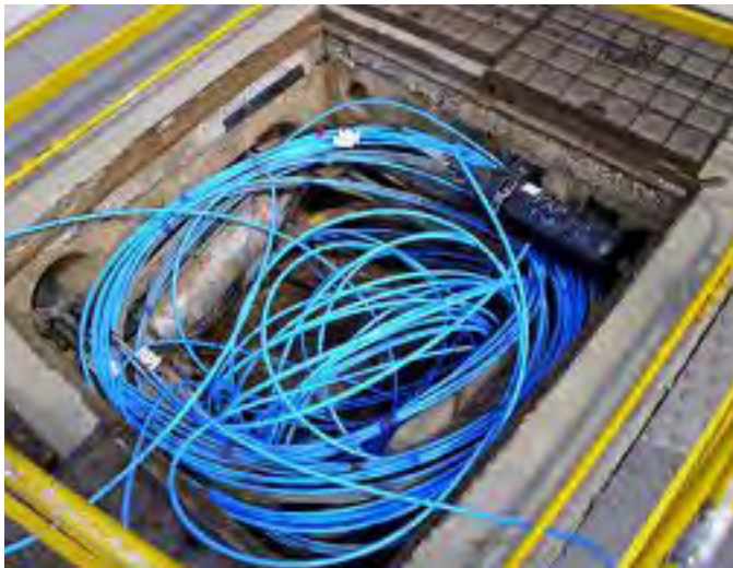
Fiber Optic Cabling (6)
