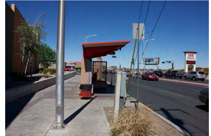
Transit shelter, light poles and other infrastructure outside of clear sidewalk area.
