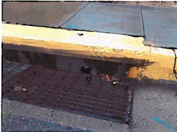
Curb inlet sampling location for outfall Y1. Curb inlet located outside the Yale Transit Facility.
