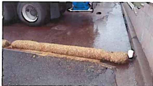
Ponding observed near Outfall PY1 and PY2.
