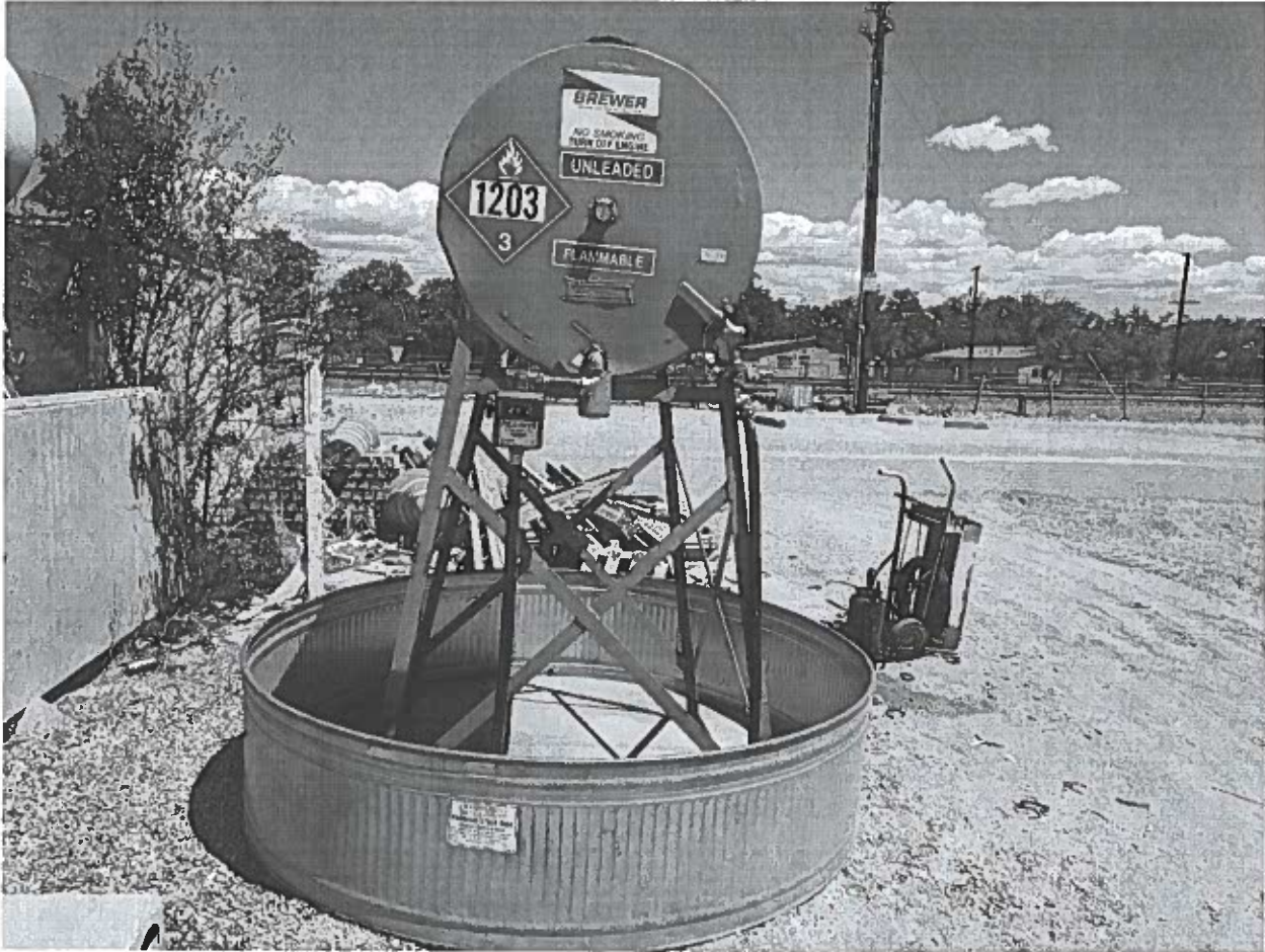
300 gallon unleaded fuel tank – Front view
